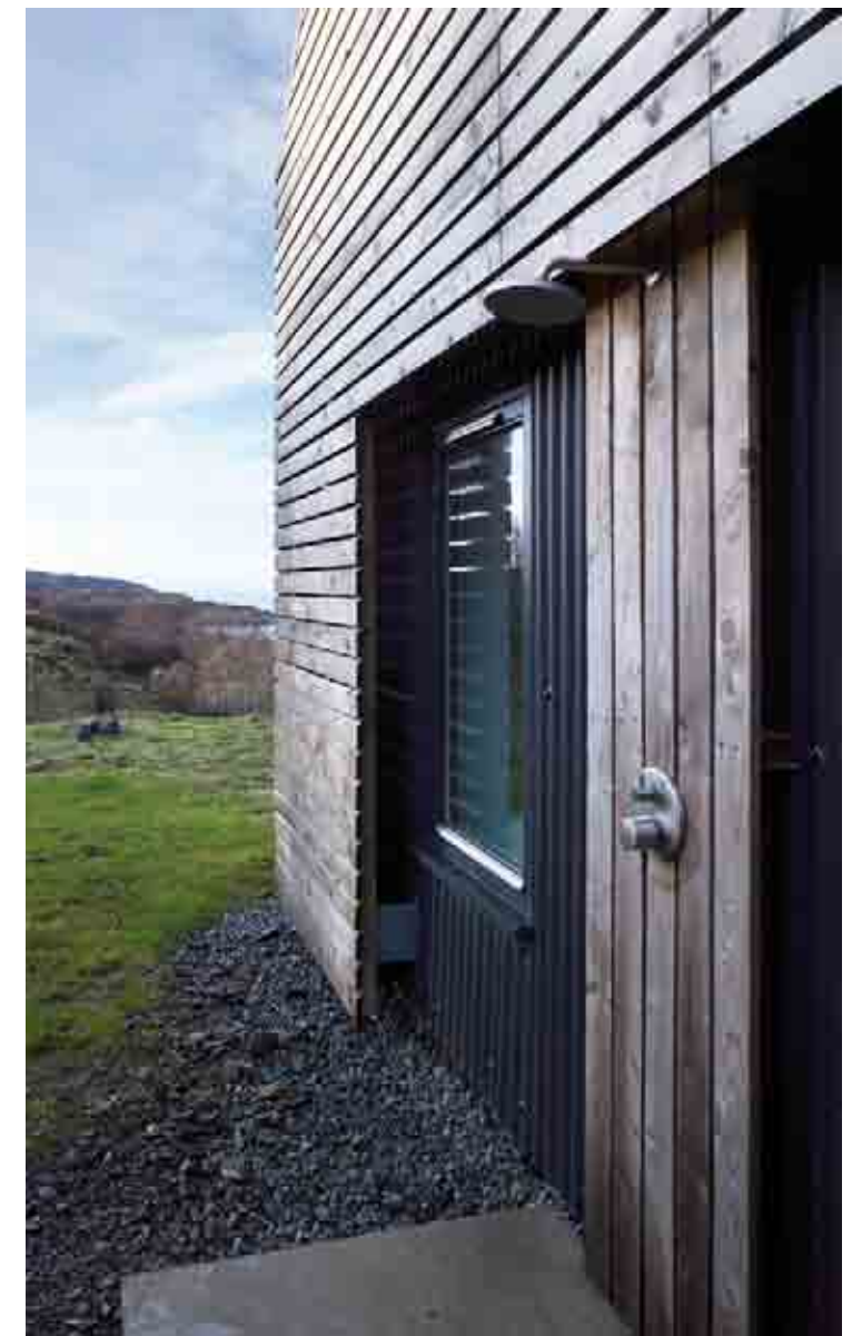
Part of the façade with corrugated fibre cement sheets is revealed at the south gable.
